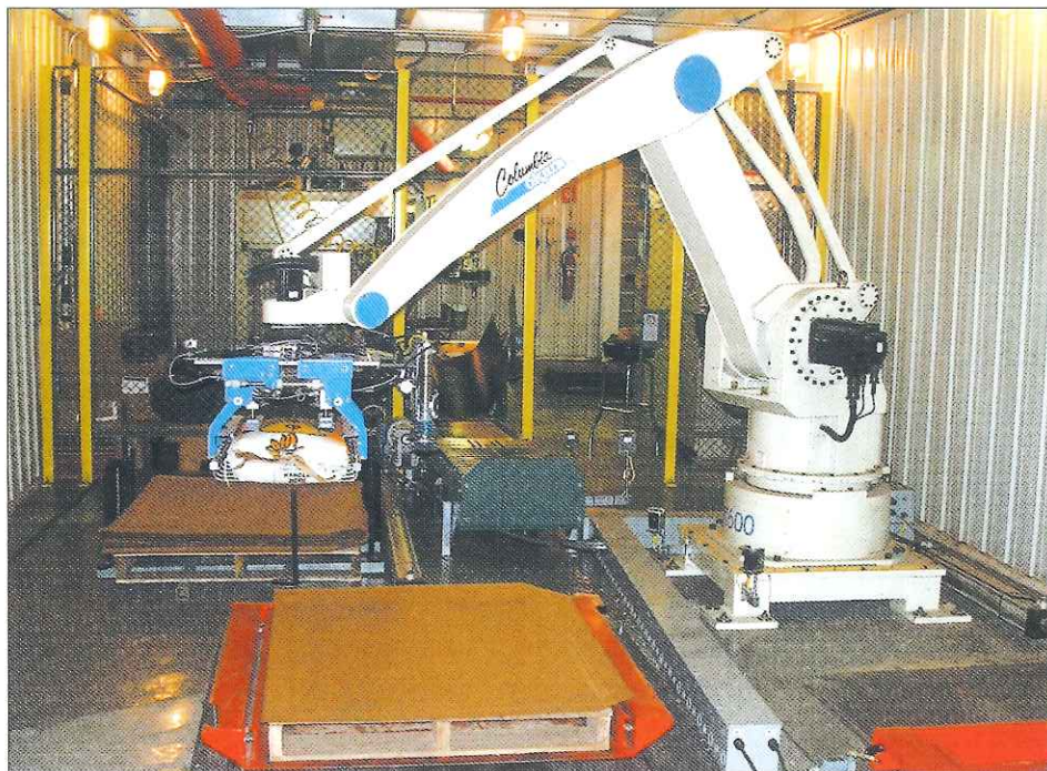
Renk Seed Company installed a Columbia/Okura LLC Model A1600 robotic palletizer in the same area where two workers had previously manually stacked bags of corn and soybean seed. A safety screen separates the packaging area from the palletizer. (Brett Renk phot)
